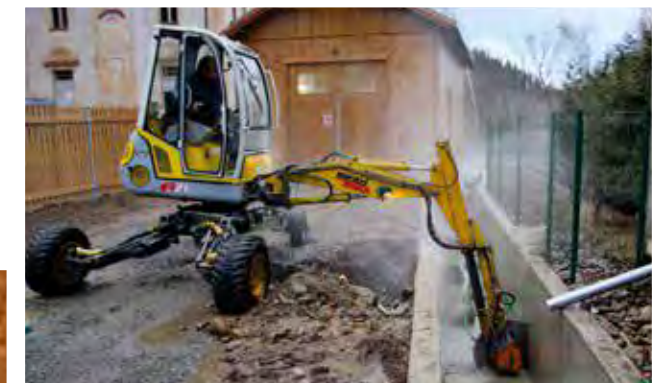
🕒 Echidna D1 diamond rocksaw cutting expansion slot in reinforced concrete water channel. (Stachy, Czech Republic)
