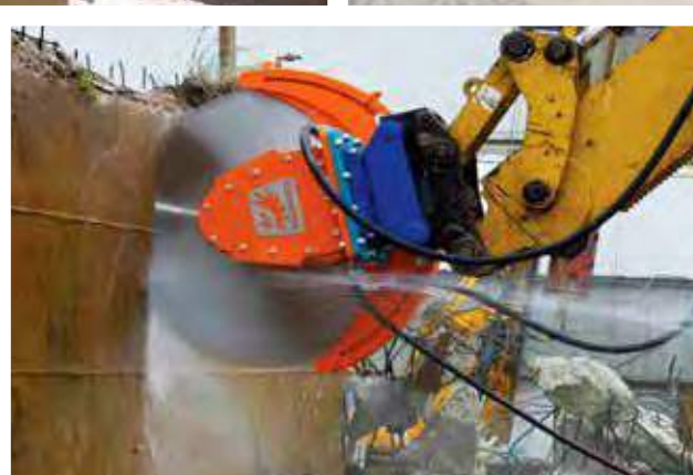
📍 High speed D4HS diamond rocksaw used for demolition of hard, reinforced concrete. (Czech Republic)
